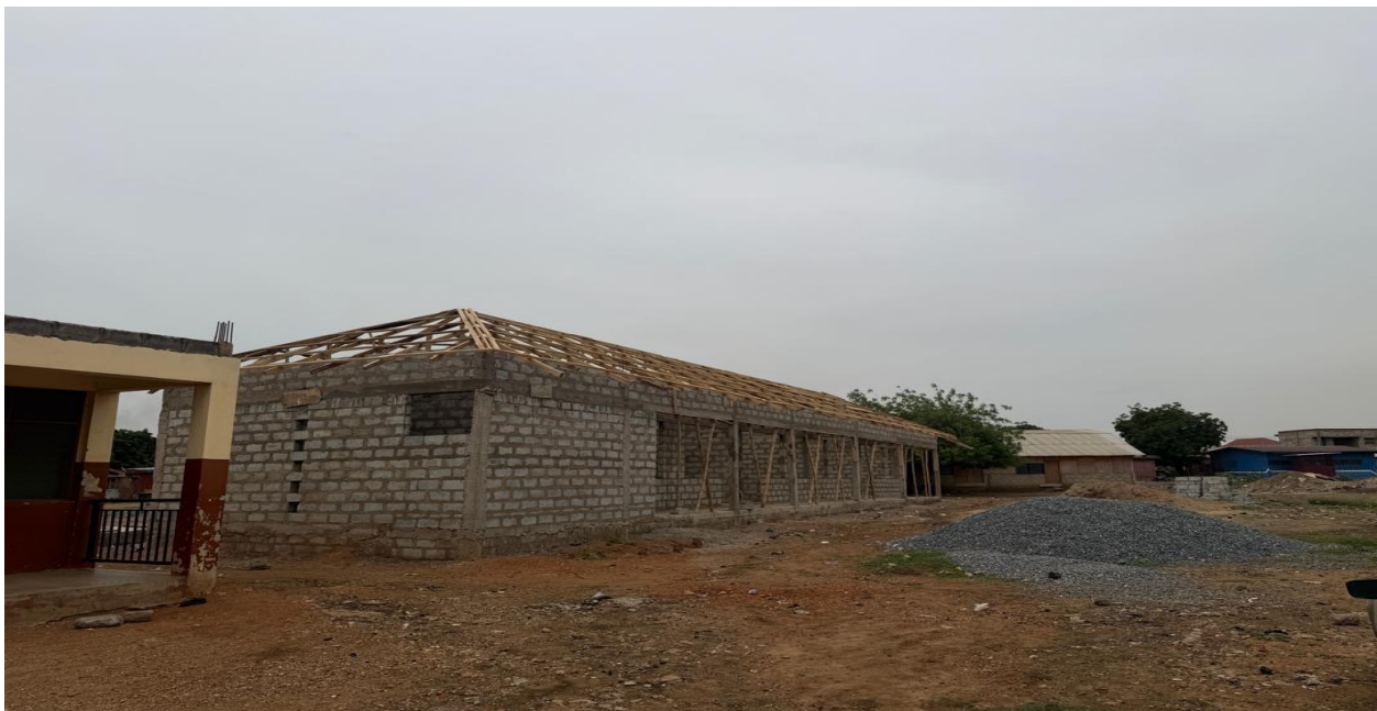
CONSTRUCTION OF 3UNIT KINDERGARTEN BLOCK WITH ANCILLIARY FACILITY AT HAANA 60% completed. All block work done, roofing members are being laid on the structure.
