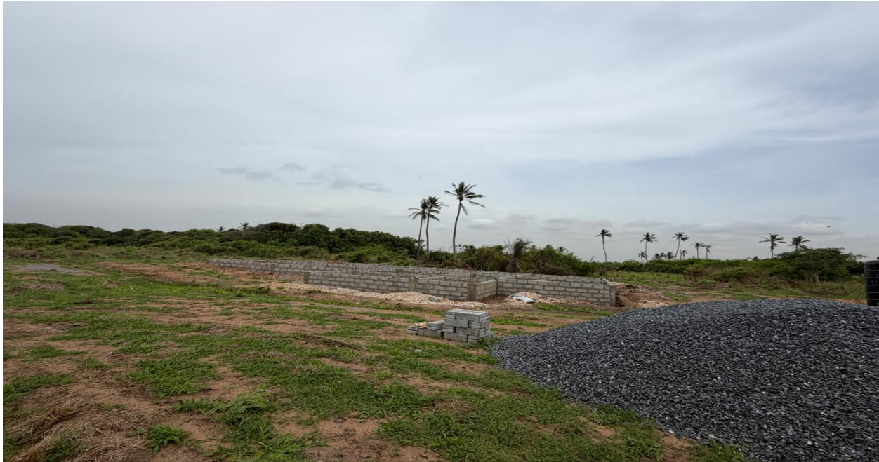
CONSTRUCTION OF 1NO. COMMUNITY-BASED HEALTH PLANNING AND SERVICES (CHPS) COMPOUND (CLINICAL SERVICES BLOCK) AT KPOI ETE 15% Completed. Block work for substructure done. Hardcore filling is yet to commence.
